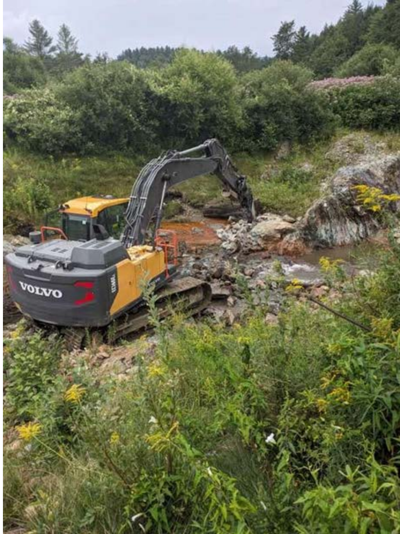
Figure 6. Excavator removing remaining portion of the dam in August 2024. Photo source: FCNRCD
